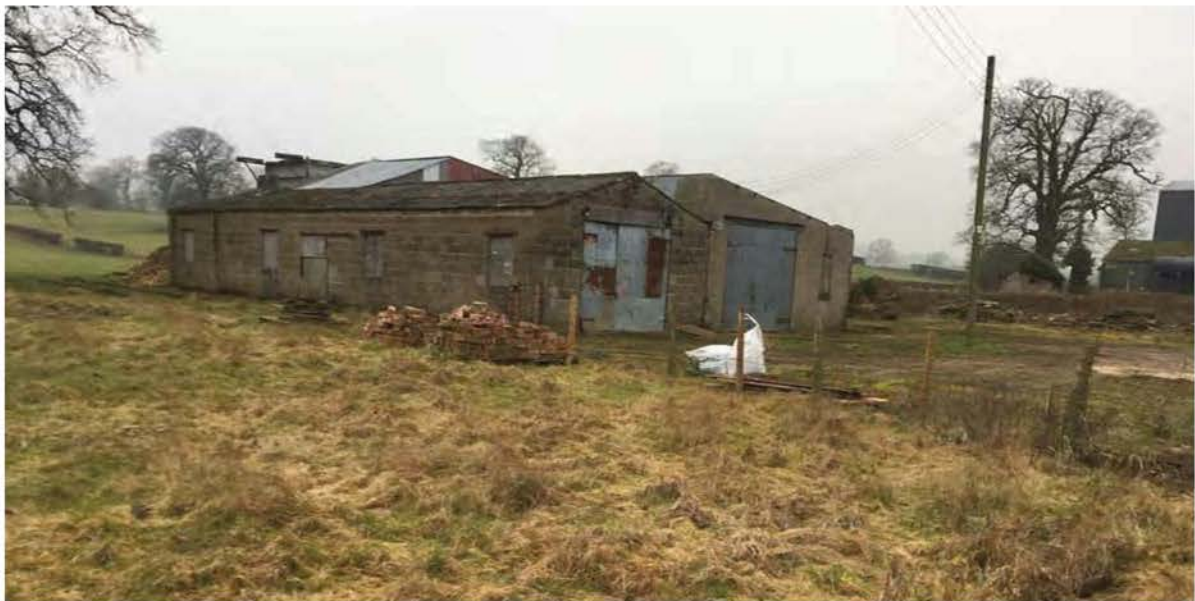
View looking south west, from the northern boundary, of the larger structure. Potential asbestos has been identified in the roof of the structure. Overhead line services seen running into the building.
